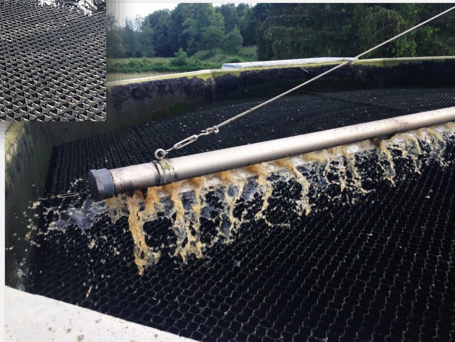
Wastewater treatment plant of CORMATIN 1 000 population equivalent View of the trickling filter with water distribution
