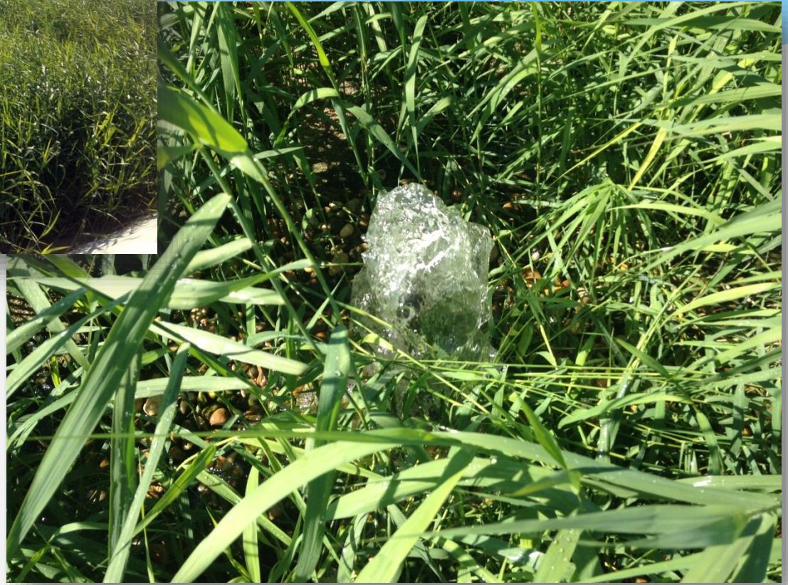
Wastewater treatment plant of CORMATIN – 1 000 population equivalent View of the second stage
