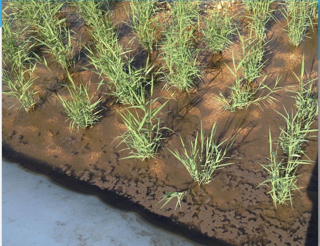
Wastewater treatment plant of CORMATIN – 1 000 population equivalent View of the first stage with flocculated sludge
